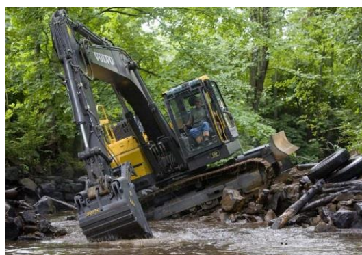
The demolition of Clark Bros. Dam on the Quinnipiac River in Southington.
